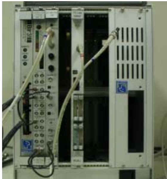
Figure 4-7 TTC system setup photo for the development of TGC electronics
